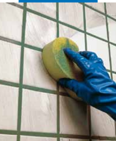
Cleaning and finishing the tile joints on a wall with a sponge
